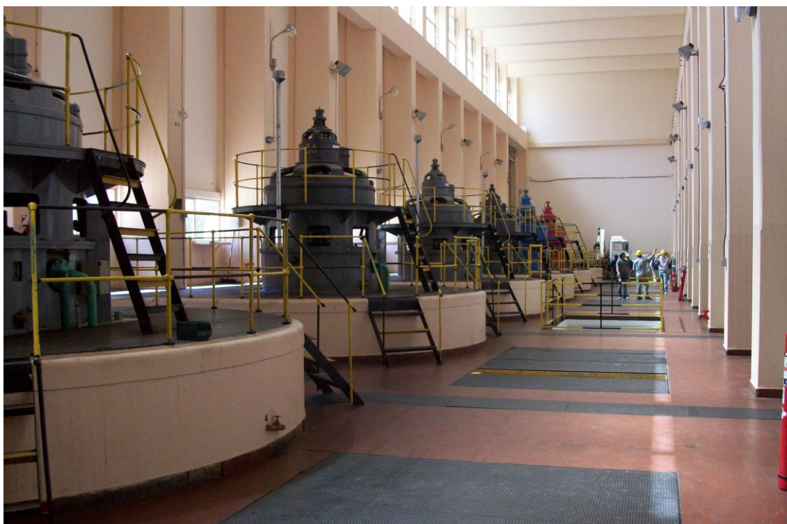
Fig. 13 Turbine row at Los Nihuiles Power Station in Mendoza, Argentina
